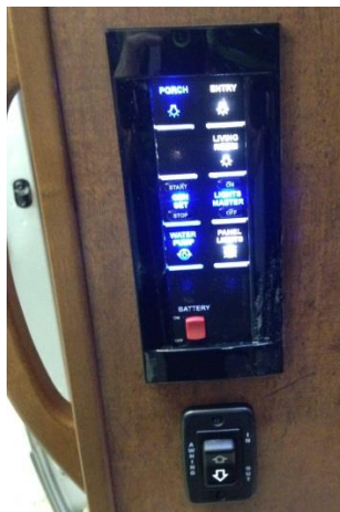
Kitchen End Switch Panel
