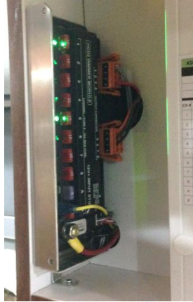
Kitchen upper fuse panel
