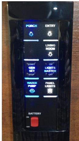
Kitchen End Switch Panel
