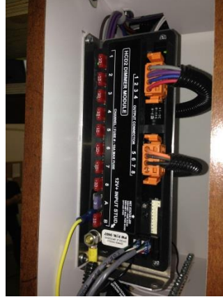
Kitchen upper fuse panel
