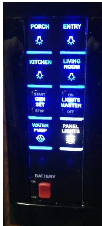
Kitchen End Switch Panel
