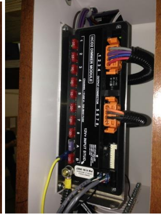
Kitchen upper fuse panel
