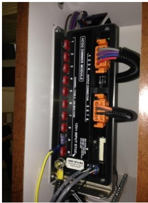
Kitchen upper fuse panel
