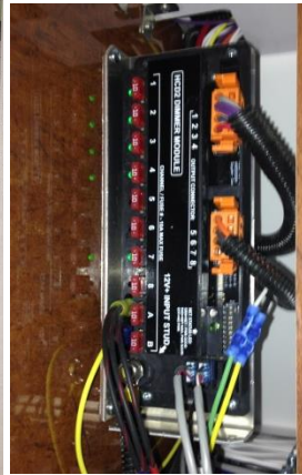
Kitchen upper fuse panel
